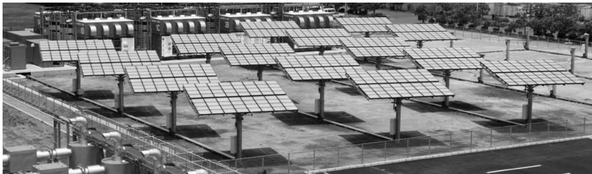
Photo 1. CPV system at Yokohama Works
